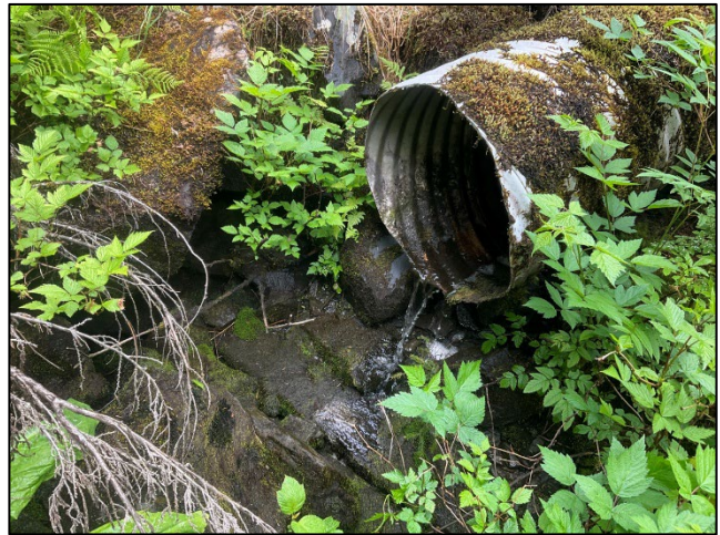
Figure 3.—Perched pipe outlet at waypoint 68.
